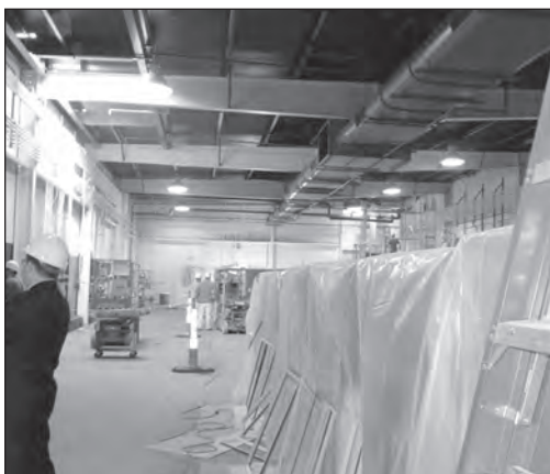
Photo: Future home of the Fabrication and Welding Technology lab in the Mary Ann Lee Technology Center.
