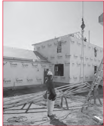
Photo: Carpentry students working with a crane to set the roof trusses.
