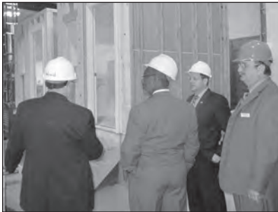
Photo: John Wood, vice president for student success, explains how INT students build a mock home from the foundation up.
